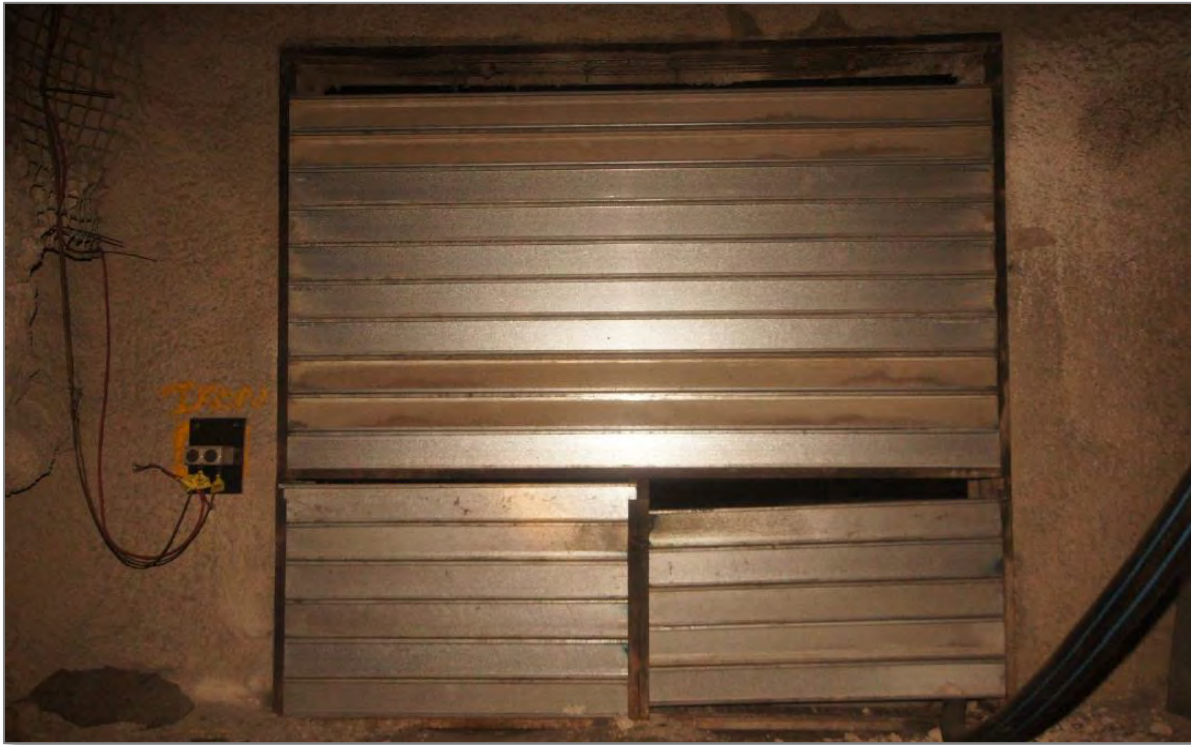
FIGURE 3-45 | TYPICAL DROP BOARD REGULATOR INSTALLED UNDERGROUND (ANGAS ZINC MINE, TERRAMIN)
