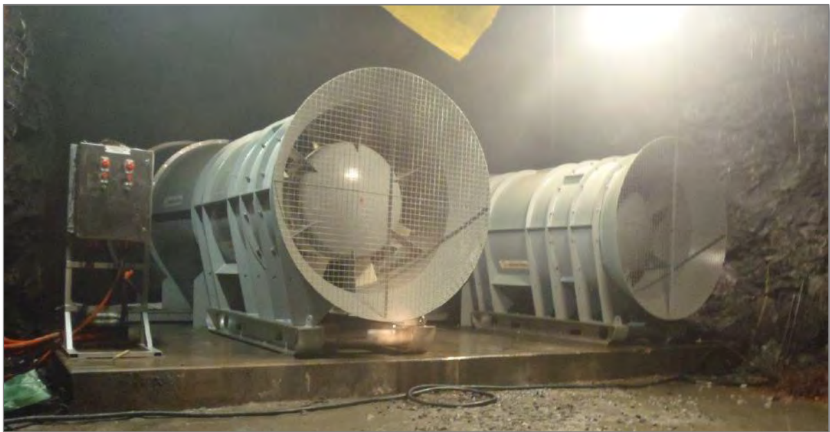
FIGURE 3-44 | TYPICAL UNDERGROUND PRIMARY VENTILATION FANS INSTALLATION PROPOSED FOR BIH (APPENDIX MV). NOTE: SILENCER WILL BE ADDED TO DAMPEN NOISE LEVELS.
