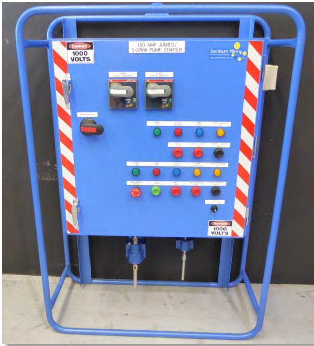
FIGURE 3-87 | EXAMPLE OF A JUMBO STARTER AND PUMP STARTER BOX USED UNDERGROUND
