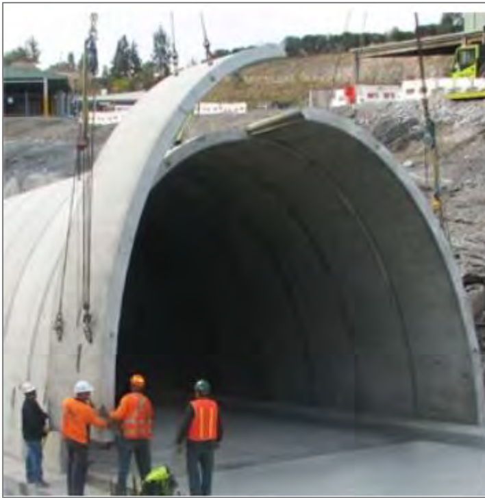
FIGURE 3-32 | EXAMPLE OF A TYPICAL INSTALLATION OF PRE-CAST TUNNELS USED IN MINING (HUMES, 2015)
