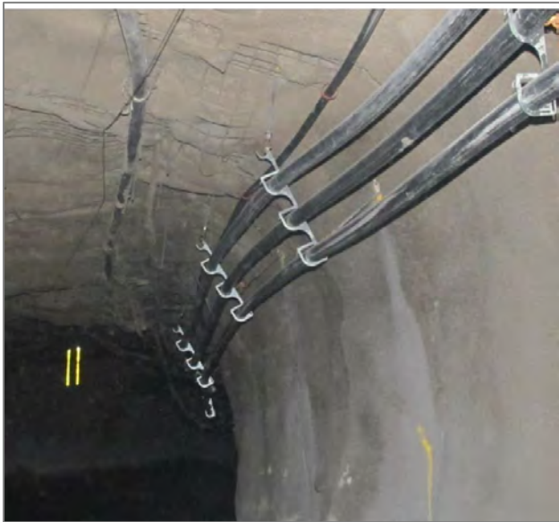
FIGURE 3-98 | POLY CLIPS FOR HOUSEKEEPING OF UNDERGROUND POLY LINES (SSORRICH, 2016).
