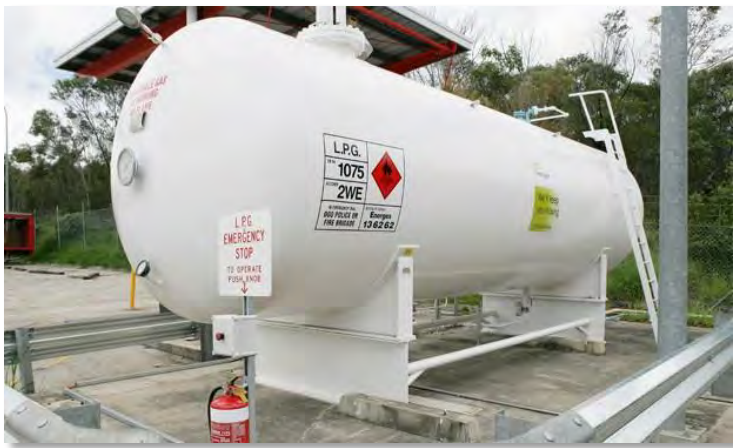
FIGURE 3-161 | STORAGE OF LPG FOR SITE USE (HOT WATER) (SAFE WORK AUSTRALIA, 2017)
