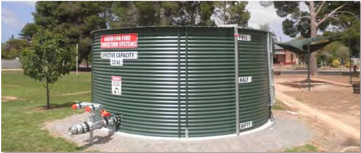
FIGURE 3-191 | EXAMPLE OF A FIRE WATER TANK
