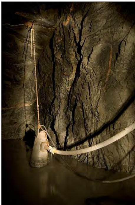
FIGURE 3-97 | TYPICAL SUMP PUMP SET UP IN AN UNDERGROUND MINE (GETTI IMAGES, 2017)
