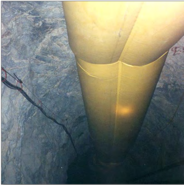
FIGURE 3-42 | EXAMPLE OF A TWIN FLEXIBLE DUCTING INSTALLATION USED IN MINING (ROCVENT INC., 2017)
