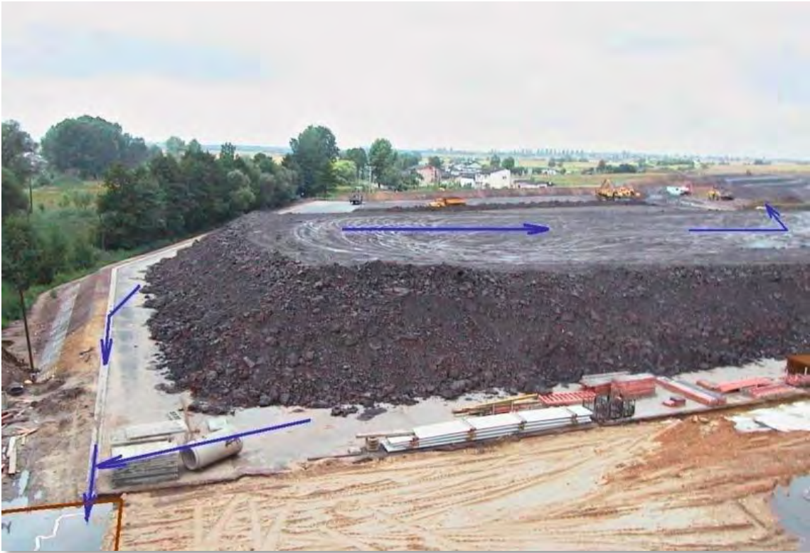
FIGURE 3-128 | EXAMPLE OF A SUITABLE STOCKPILE LAYOUT SHOWING DIRECTION OF FLOW FOR WATER RUN-OFF. (ZIEGELINDUSTRIE INTERNATIONAL BRICK AND TILE INDUSTRY INTERNATIONAL, 2011)
