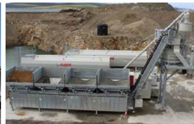
Concrete batching plant
