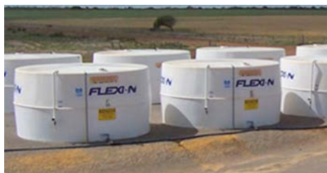
Water treatment tanks
